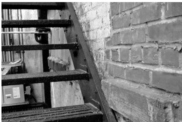
Triangle today: Ninth floor fire escape today. In 1911, workers had to climb out a window to get to the fire escape, which ended two floors above the street. The original window ledge and opening can be seen filled with brick.
